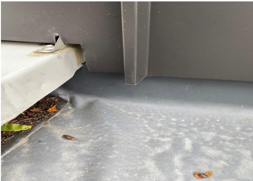
Figure 7. Membrane in sole of gutter appears deteriorated compared to upstand. Material 1.1mm, Age approx. 3 years.
