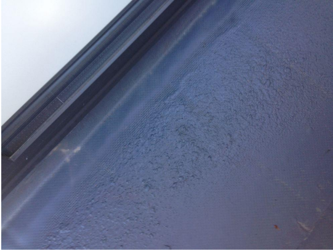
Figure 8. Membrane blistering from heat from upstand reflection. Material 1.2mm, Age approx. 4 years
